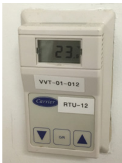
Typical Existing Thermostat
