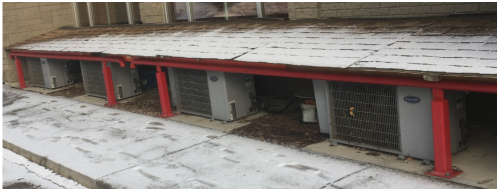
Four of the eight air conditioner units along south side of building
