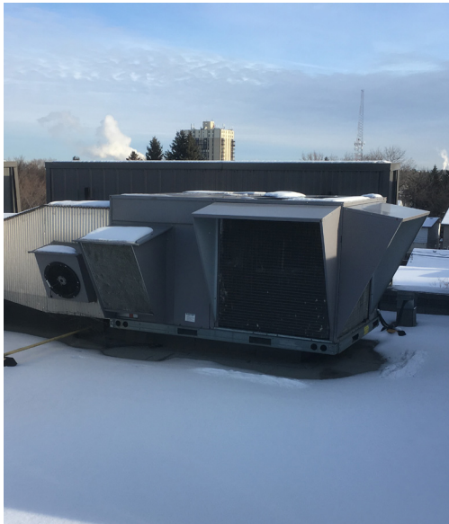
RTU-15, manufactured in 2009, located on Phase 2 roof
