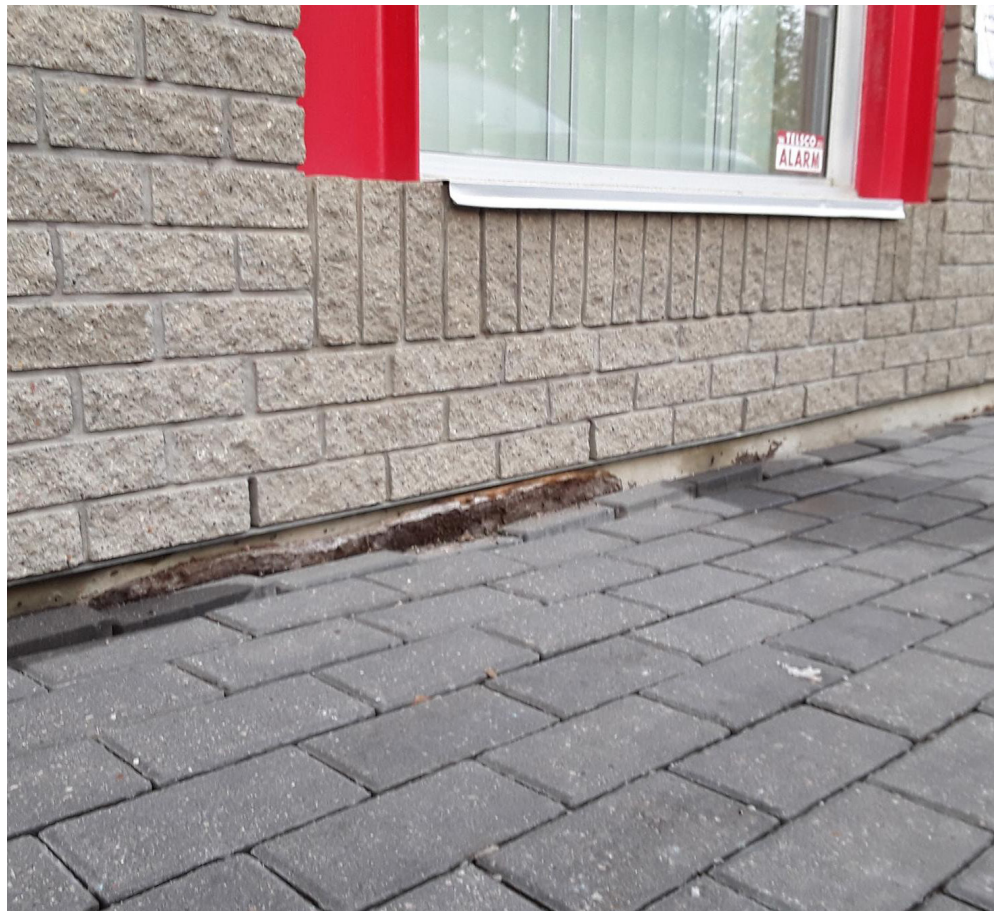
Image: Damaged insulation at exterior wall base.
