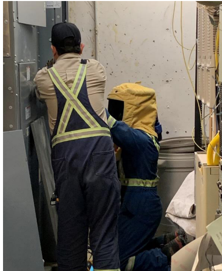
Data Logger Installation - 29 January 2020
