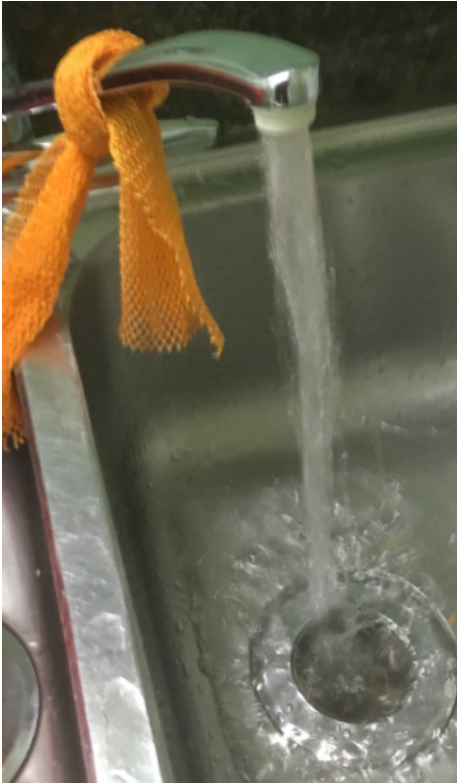
Kitchen sink without aerator
