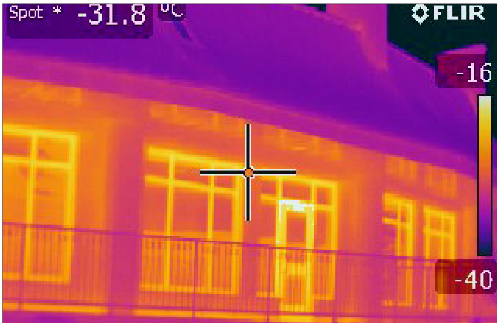
Image: Thermal Camera Showing Heat Escaping
