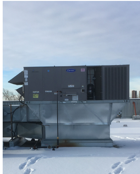
RTU-6, manufactured in 2018, located on Phase I roof
