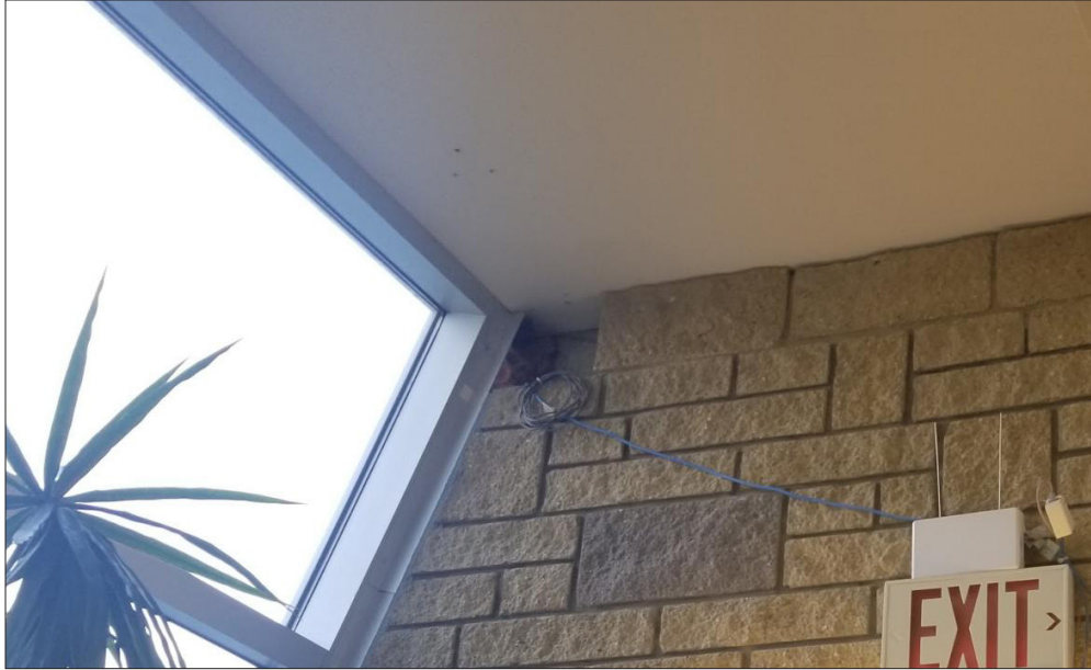
Image: Interior Wall where Hole was Found
