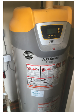
Phase 2 water tank
