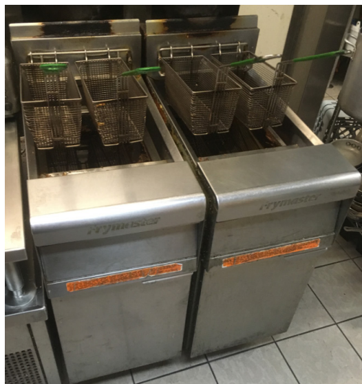
Commercial kitchen natural-gas deep-fryers
