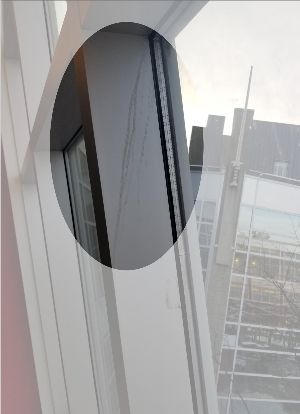
Image: Leaky Window
