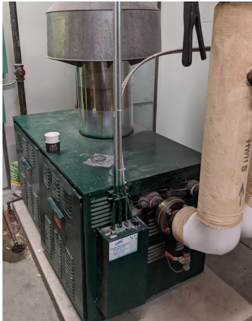
Phase I boiler
