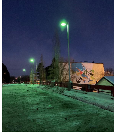
Parking Lot Pole Luminaires (Metal Halide Lamping)
