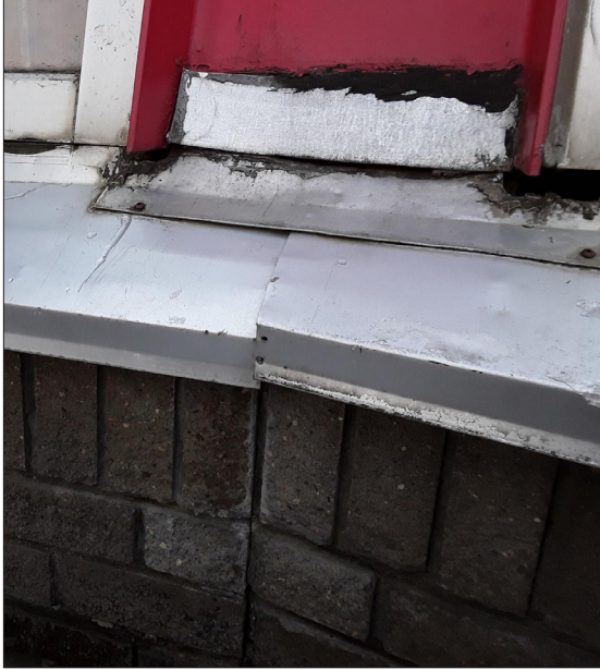
Image: Flashing Damage
