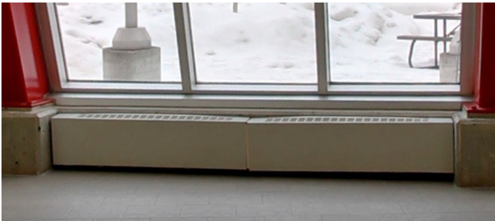
Radiator terminal units for heating curved hallway
