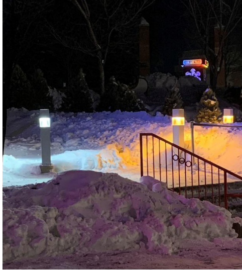
Exterior Bollards (note the two illumination colours – HPS and Metal Halide or Colour Corrected HPS)
